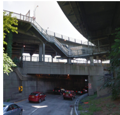
Say goodbye to these stairs on the George Washington Bridge path... in ten years. Photo: Google Maps
